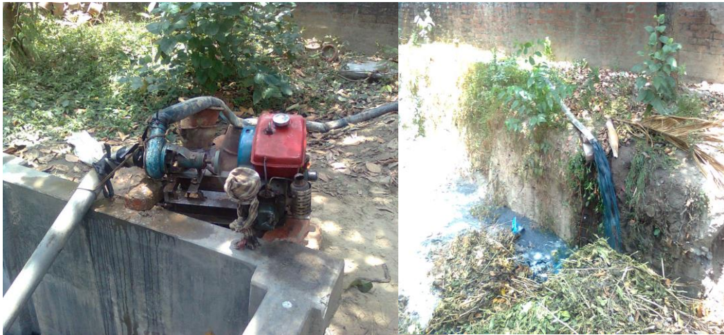
Fig. 2: Disposal of effluent from storage tank
