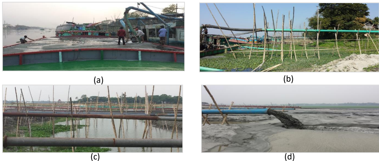
Fig. 1. Hydraulic filling procedure (a) dredged fill transported by barge (b) & (c) dredged fill transferred to the site in the form of slurry and (d) delivery of fill to the site.
