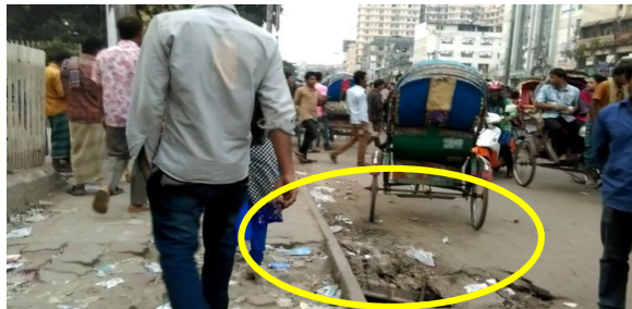
Poor Quality of Walkway (New Market area)
