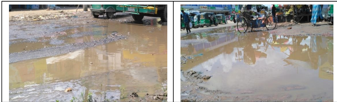
Fig. 1: Damaged & Water Logged Areas at Pahartali, Raozan, Chittagong.
