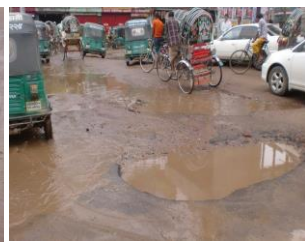
Fig. 11: Bad effect of overflow on road (Location: Bahaddarhat)
