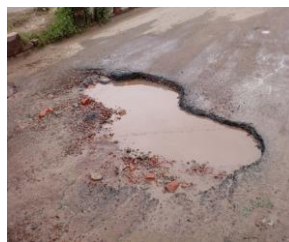
Fig. 10: Road damaged due to water logging (Location: Muradpur)
