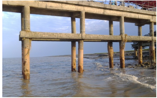
Photo:4 Damaged BIWTA jetty near shoreline at Sandwip (September, 2014)
