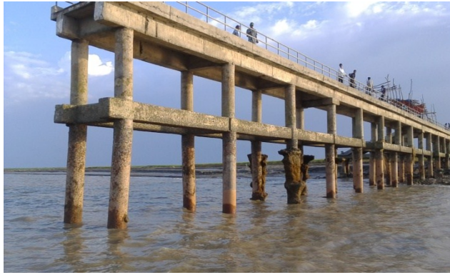
Photo:3 Damaged BIWTA jetty at Sandwip side low tide (September, 2014)
